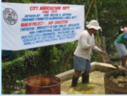
Personnel loading animal waste into the inlet of the 50 cubic meter biogas digester facility located at the City Nursery
